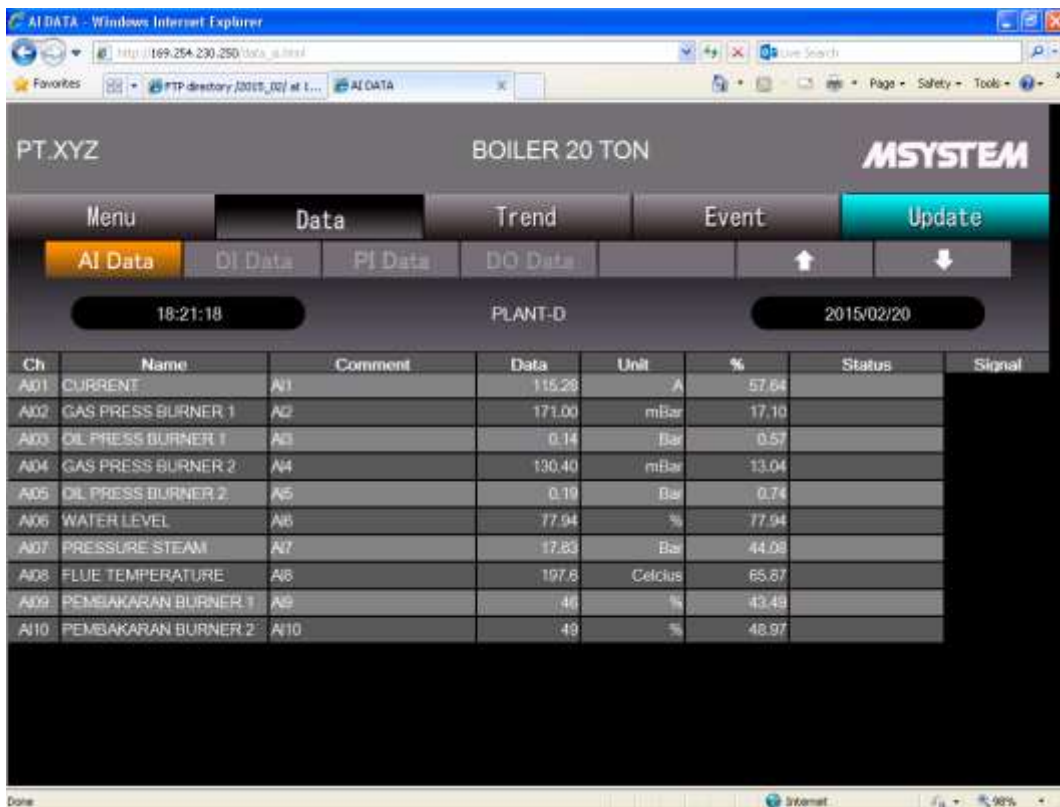
Fig. 10. Overview of PC Display for Remote Access Control (Analog Input).
